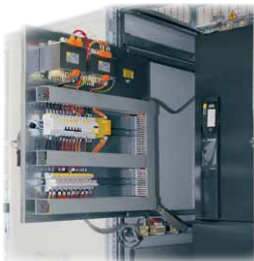
Detail of the auxiliary circuit plate (left-opening panel).
